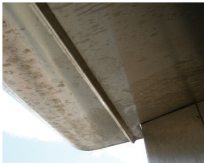
Fig. 4. Stainless steel cladding that could not be cleaned by frequent rain showers.
