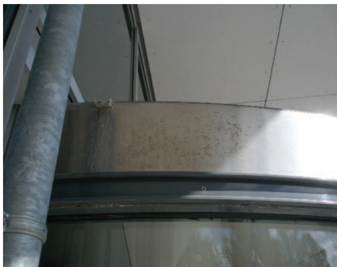
Fig. 3. Close up of Fig. 2 which shows corrosion due to aerosols.
