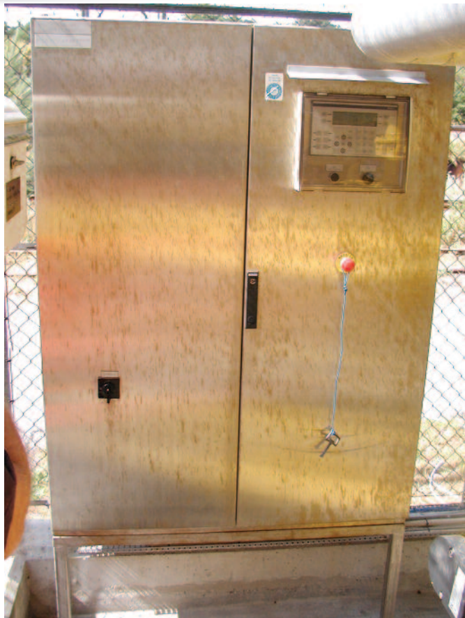
Fig. 8. Flash rust on switchboard cabinet made from 316 steel caused by aerosols from the sea.
